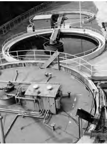
As Norwich grows, wastewater treatment infrastructure, such as the clarifying tanks shown above, will need to be expanded to accommodate increased flows.
